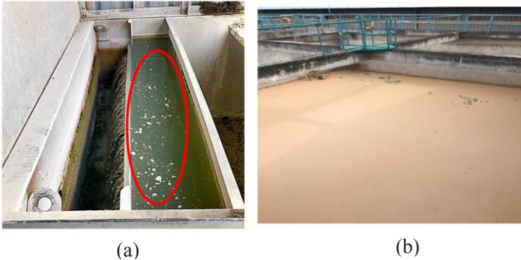
Figure 1: Problems faced (a) Suspended solids carry-over due to thick sludge accumulation at the dissolved air Flotation tank. (b) Poor settling of sludge at sequential batch reactor tank prior to discharge.
