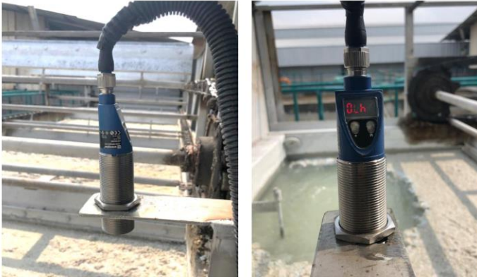
Figure 3: Ultrasonic level sensor installed on top of the dissolved air floatation tank.
